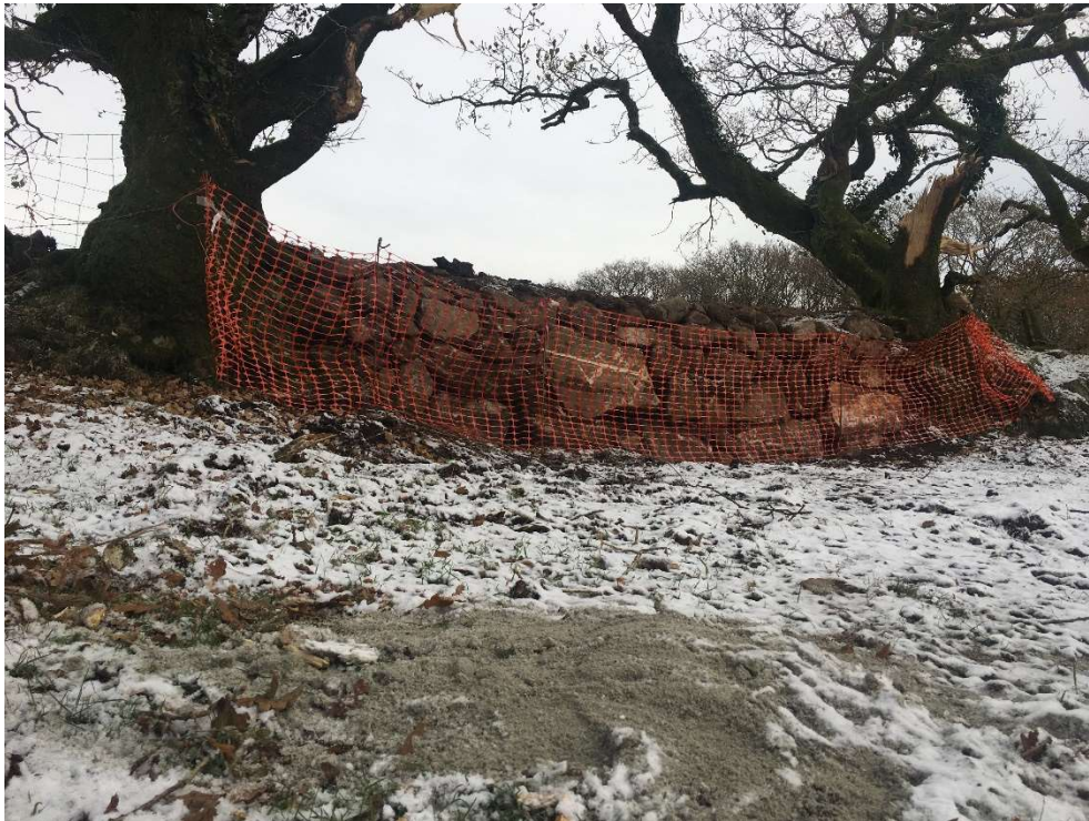
Figure 25: Workings but with no associated evidence of pollution on the western side of rebuilt wall adjoining field above Tin Park recorded by Tony Hawkins 1010h 14Dec22
